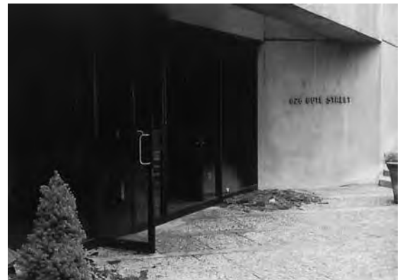
The detonation blew out exterior windows on the building's main floor.
