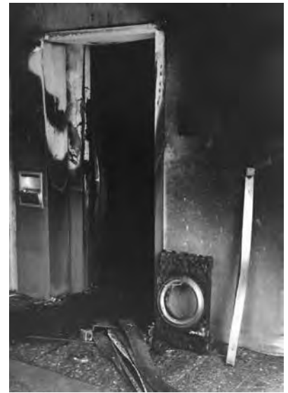
An incendiary device that exploded in the Institute's elevator in August 1980 caused extensive damage.
